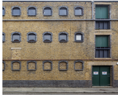
Swan Wharf: In nearby Fish Island, the interest of the facade is achieved through the repetition of evenly spaced openings with blue brick reveals; modest in scale but generous in number.
